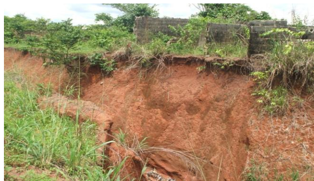
PLATE 3: Gully Erosion Site at Nekede (Authors fieldwork, 2016)
