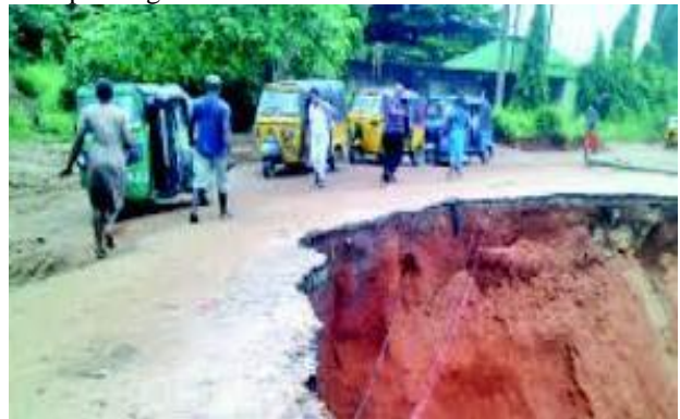
PLATE 2: Gully along Nekede Road (source: Nairaland forum, 2016)
